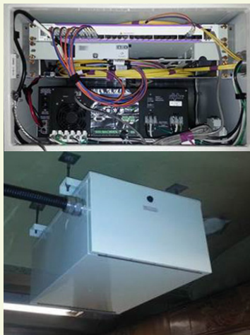
Alpha's Ceiling Mount Backup Power Solution at an underground subway station in NYC
